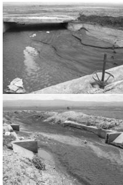
Fig. 6. Soil sedimentation in main canal (above) and division box (below).
